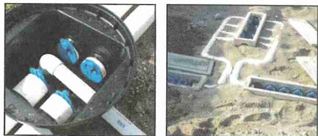
Custom Distribution Boxes with Equalizers installed
